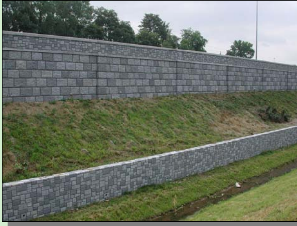
Concrete Formliner in a Stone Pattern on a Sound Barrier and Retaining Wall along Canal Parkway in Allegany County
