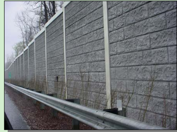
Sound Barrier with a Stone Pattern Concrete Formliner Finish along I-83 near Timonium
