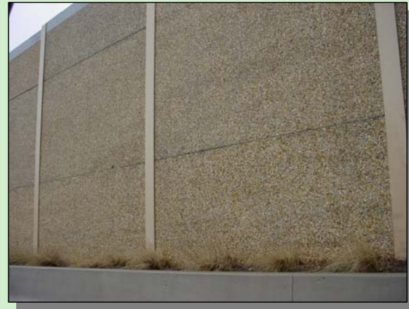
Noise Barrier with a Patterned Concrete Finish along I-95 near the I-895 Split
