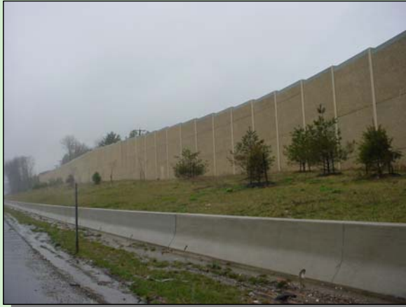
Noise Barrier with a Patterned Concrete Finish along I-95 near the I-895 Split
